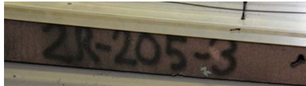
Fig. 12: Photograph of the panel identification number of the panel for documentation in the DCS.
